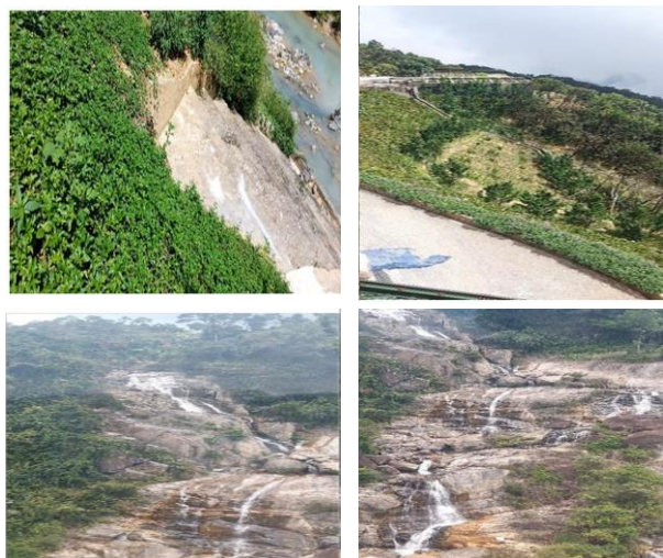
Figure 4. Ditch and drainage system at the top and foot of Ba Na tourist area
